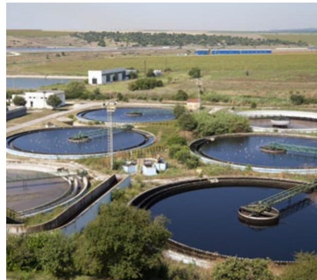
Figure 20: Sewage treatment plant
